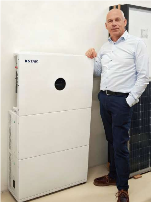
03 Residentieel ESS-project in Nederland
