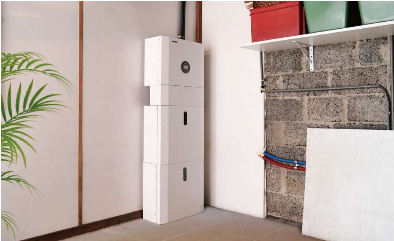
10 Residentieel ESS-project in Nederland
