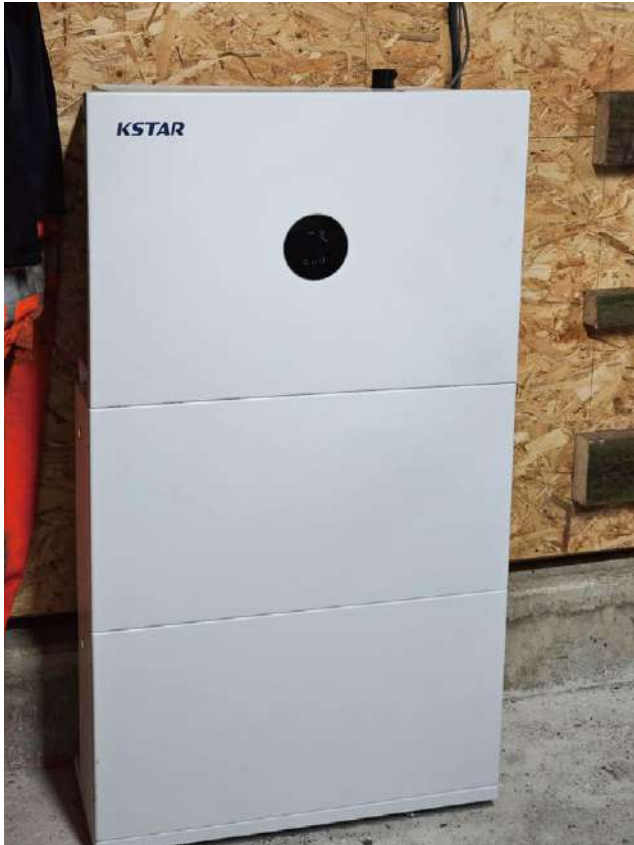
02 Residentieel ESS-project in Nederland
